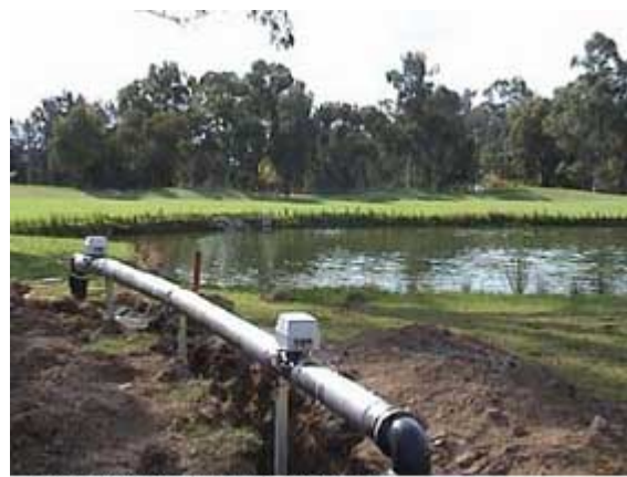
The Hydrosmart system installed on pipework at Liverpool.
