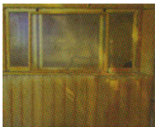
No, it's not paint - overspray with iron at 32 parts per million prior to treatment.
