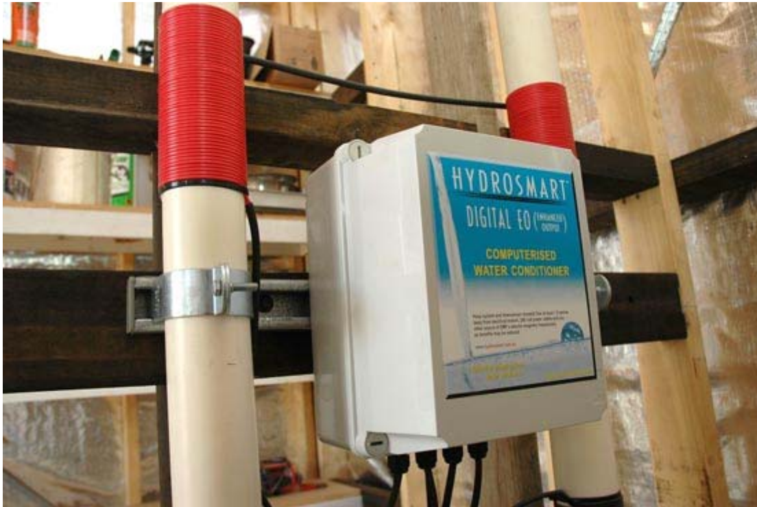
A 40 mm Hydrosmart unit installed at Pam and Brendan Drechsler's property near Bendigo.
