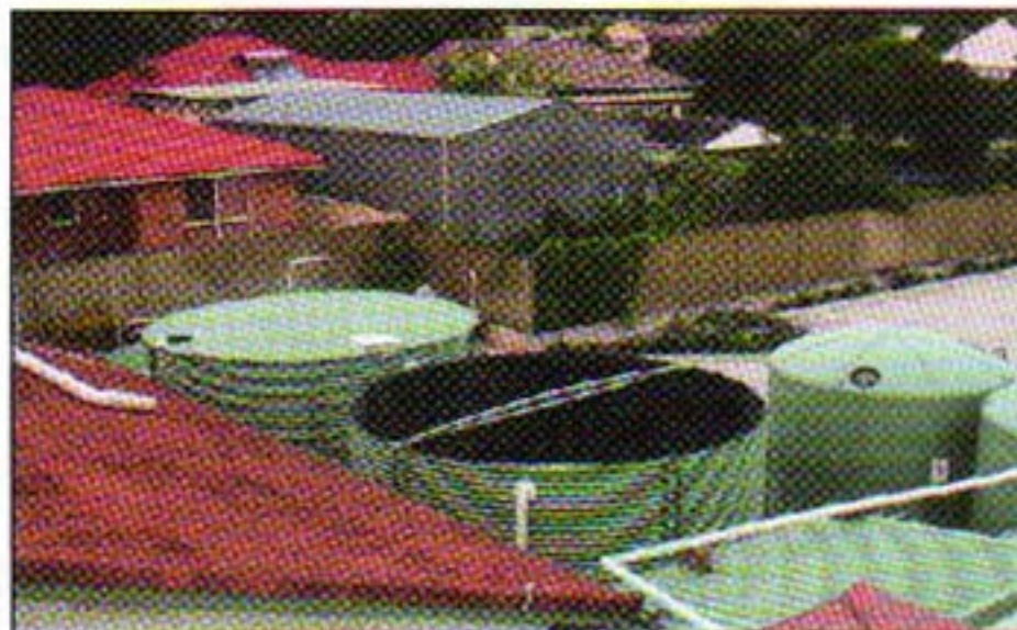
Storage tanks at Albion Park Bowling Club form an important part of the club's water management plan.
