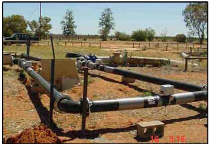
A 200mm system installed at Table Grape Growers Australia at their vineyards in Menindee NSW. Salinity ranges from 2400-3300EC with a pH up to 9.3
